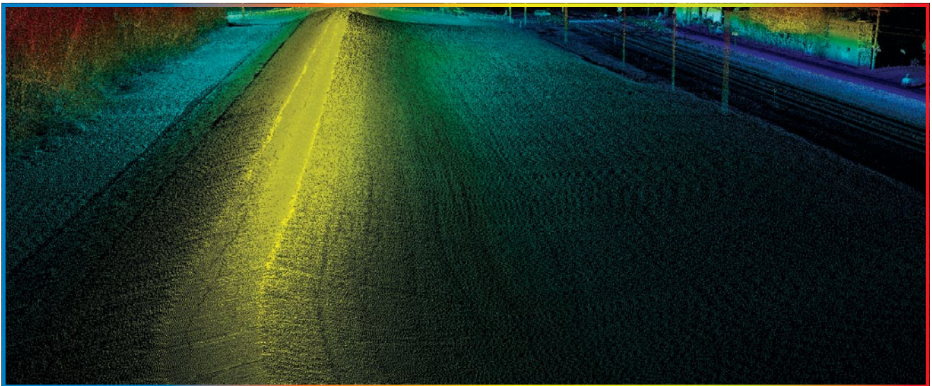
Figure 3 Crack in surface pavement of levee rendered visible after sampling data down to surface level.
