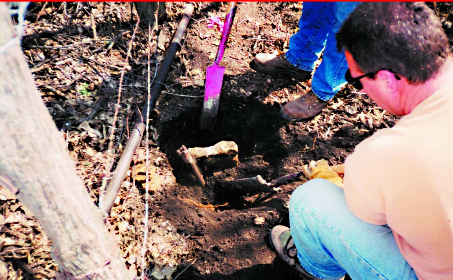
After tying out the location of the government limestone, the careful excavation of it and the witness pipe begins. The stone was lowered and a new monument was set over the top of the stone eliminating the double monument at this location.
