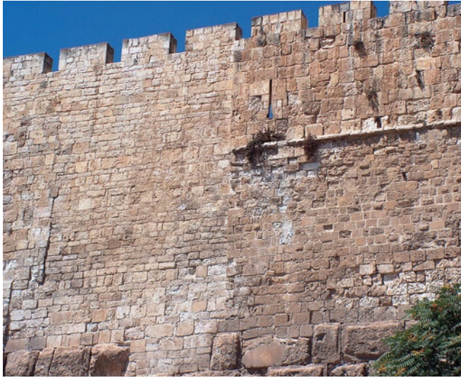
Figure 1 Eastern wall of Jerusalem's Temple Mount after earthquake-induced displacement. All images courtesy Israel Antiquities Authority and Mabat 3D Technologies Ltd.
