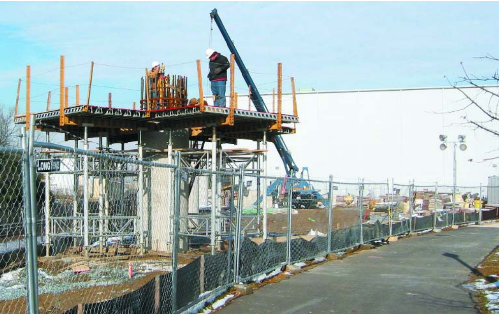
Survey control stakeout for new railroad pedestrian overpass over WMATA and CSX tracks in Silver Spring, Maryland.
